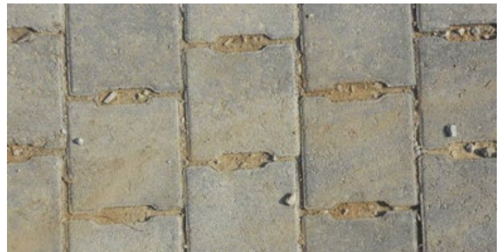
Clean permeable pavers (top) versus clogged (bottom)
