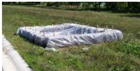
Good example of above grade system with straw bales and a polyethylene lining. A "Concrete Washout" sign should be installed at this location.
