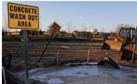
Poor job of containing washout inside of the designed area. Washout material should be removed when capacity becomes an issue.
