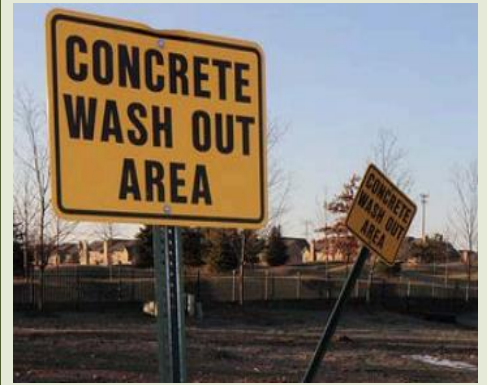
Properly identify concrete washout areas with visible signage.
