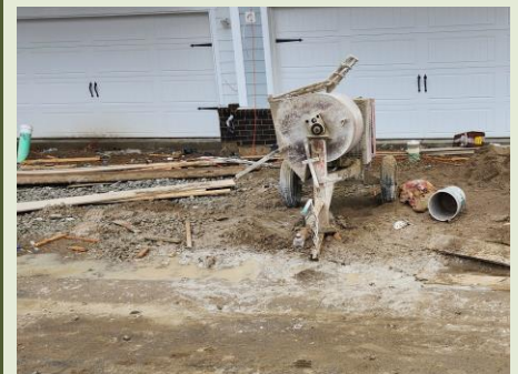
An improperly managed mortar mixing station can allow corrosive washwater to enter the stormwater system through curb inlets.
