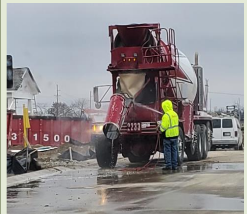
Avoid doing final rinse of trucks outside of the washout area.
