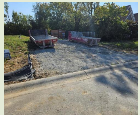
Washout area is accessible and placed on stone pad and away from storm inlets and water resources.
